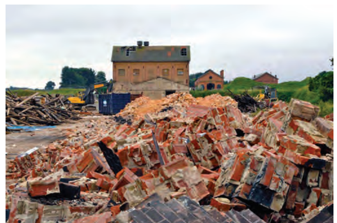
The winding house just before demolition in August 2014, with the two workshops to the rear. Photo Colin Varrall
